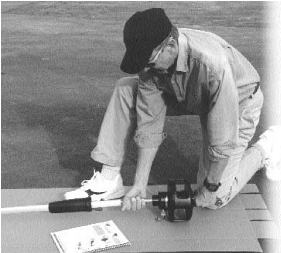
The unit design allows easy owner installation, but many people hire a rigger to do the job.
